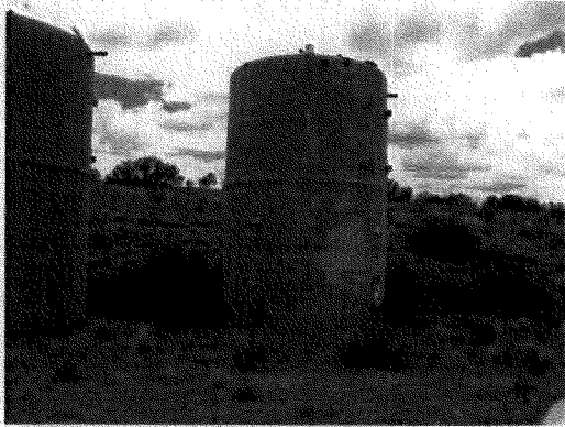
Two (2) magnesium chloride storage tanks. No longer used.
